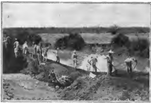
Protecting the roads from floods in the central part of the Yaqui valley, Mexico. Supplies for the American army go over these roads. (Samuel Frankel.)
